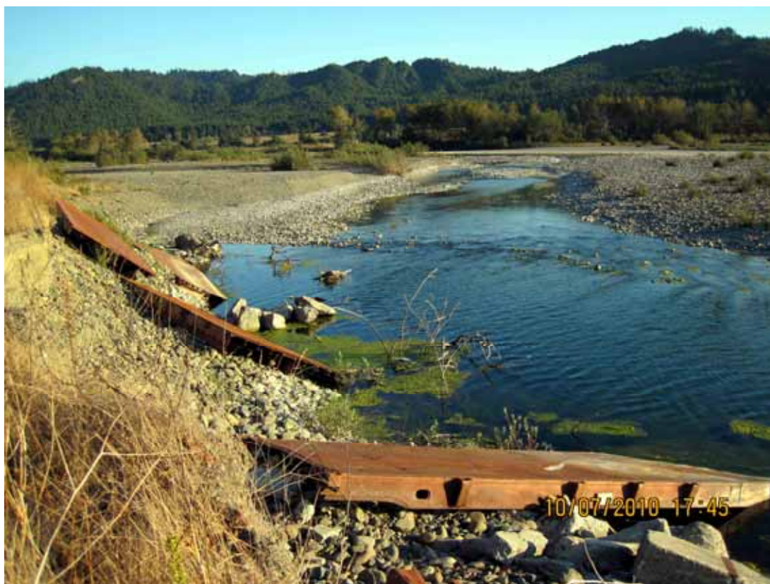
Figure 12. This photo was taken looking upstream on the mainstem Van Duzen River not far below Yager Creek. The channel is shallow and lacks pools. Low flow conditions promote stagnation. Use of old flatcars has failed to stabilize the bank. Photo by Pat Higgins.
