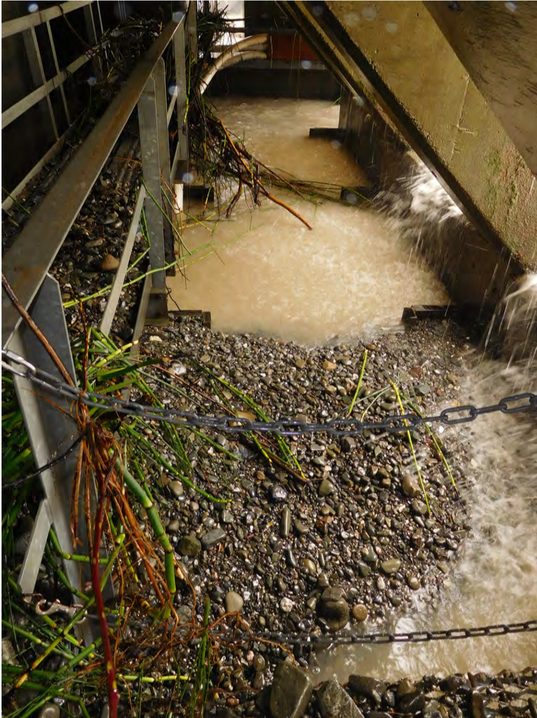
Gravel entirely obstructing the fishways in the lower portion of the 'fish hotel' structure. Fish cannot reach the fish ladder until the gravel is cleared.
