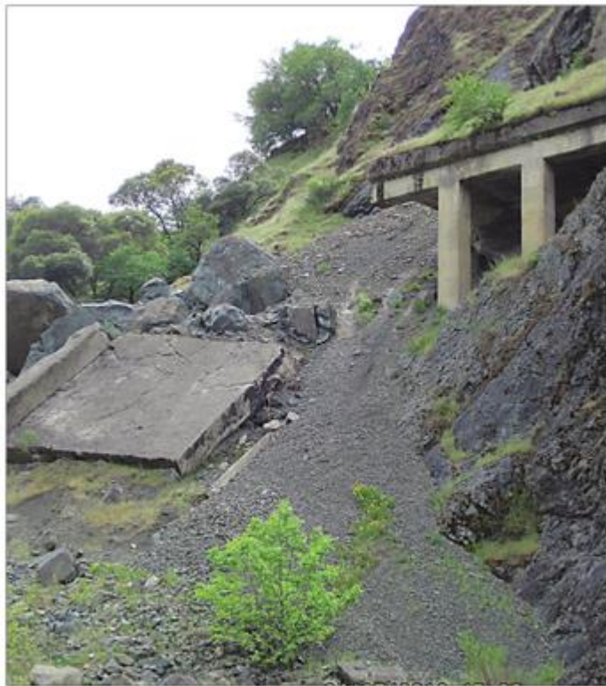
The tunnel immediately south of the Woodman Creek crossing has collapsed and been partially filled by one of many landslides exacerbated by the defunct rail line in the Eel River canyon. Photo: Scott Greacen.
